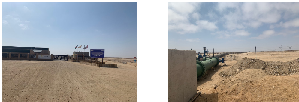
Figure 6. Arango Desalination plant
