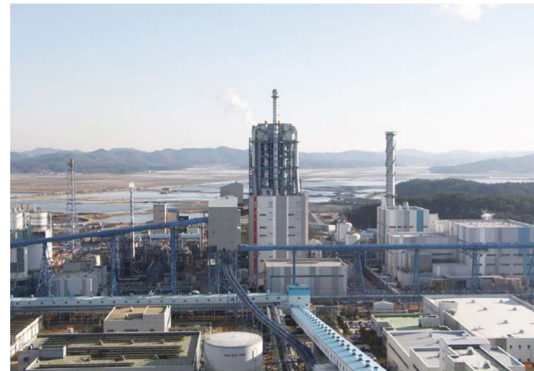
Figure 11 | A 300 MW IGCC plant in Taeon, Korea Western Power Co., Ltd Korea
