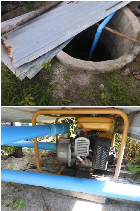
Figure 1 Typical Well and Pump (petrol pump) Installation
