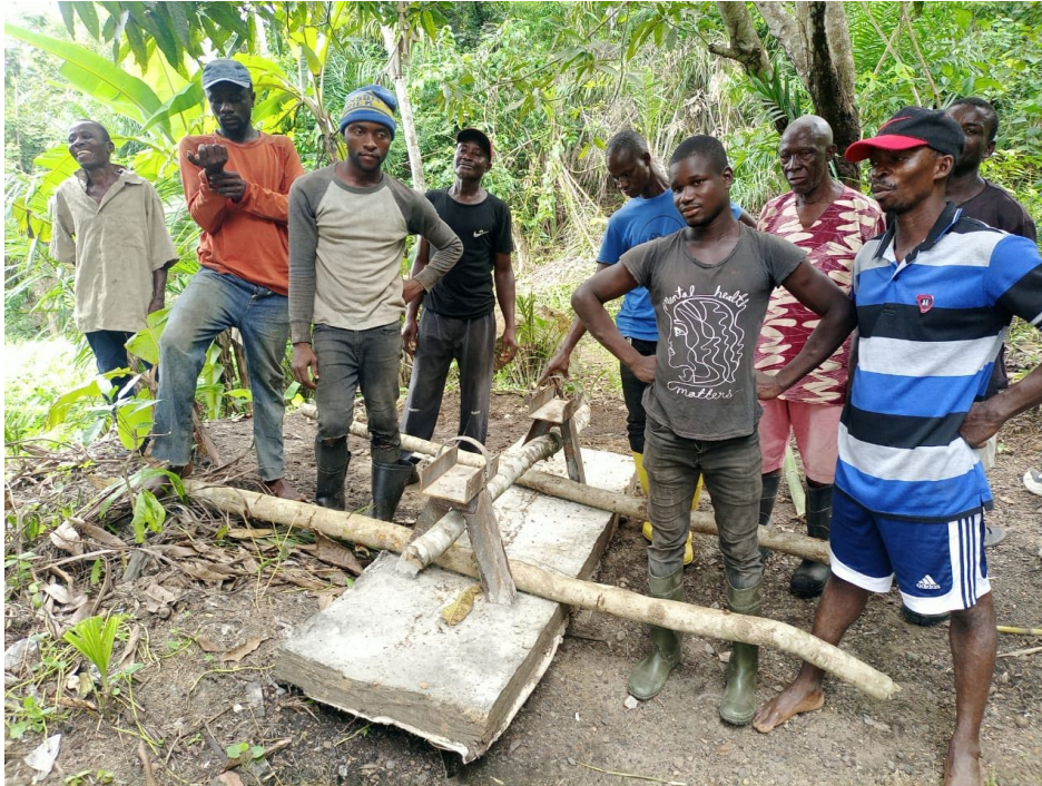
Figure 20: Solar pump mounting platform cast in concrete with two embedded metal supports, ready to be moved into pond
