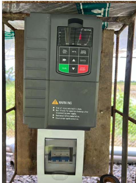
Figure 23: Support showing Controller inside security cage.
