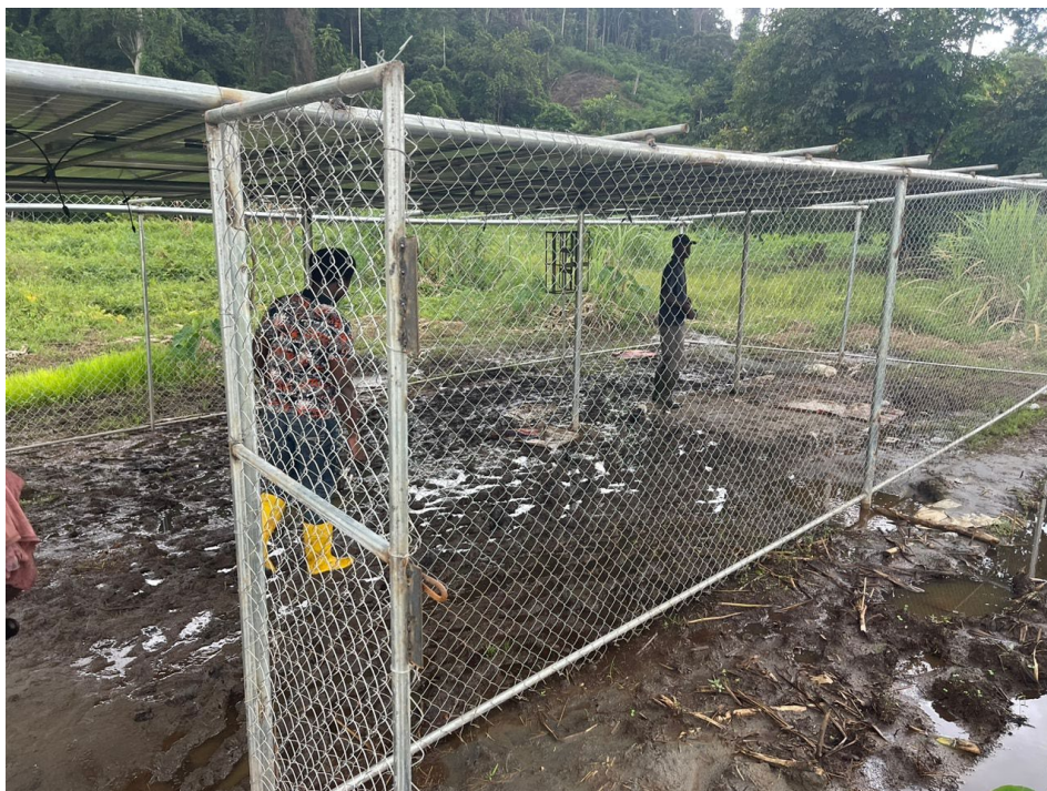
Figure 10: Installed PV Panels with fencing and gate
