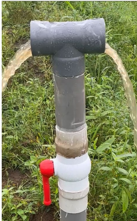
Figure 17: Irrigation Outlet with Control Valve
