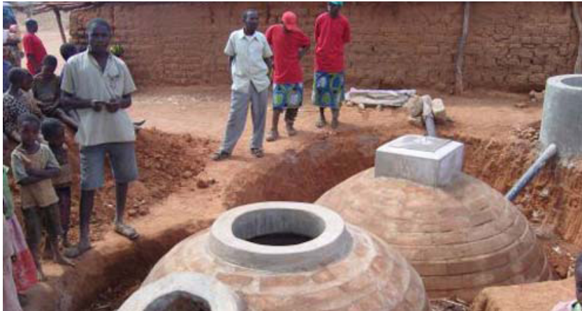
Figure 1: Top-Typical design of a double-chamber fixed dome biodigester (Model CAMARTEC, Tanzania). Bottom-Biodigester CAMARTEC built, prior to being plugged with soil (CAMARTEC, Tanzania)
