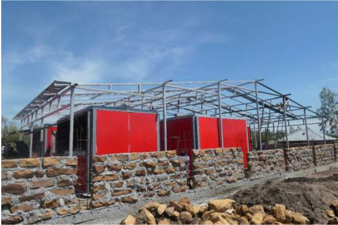
Figure 8: Peri urban site solar panel orientation and charging hub construction in progress
