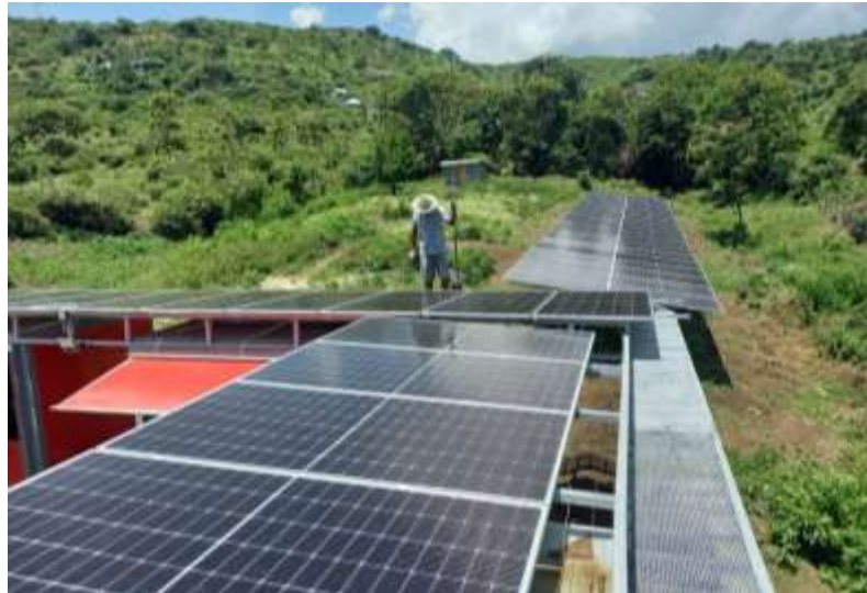
Figure 10: Rural site solar panel orientation and charging hub under development
