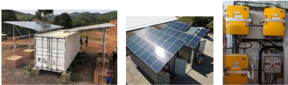
Figure 75: From left to right: Examples of two types of containerised off-grid solar systems, hybrid inverter
